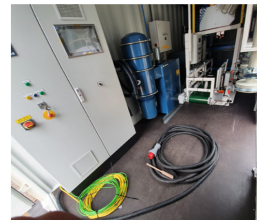
08/ Bagging line, vacuum system, PLC
