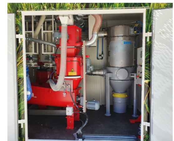
06/ Continuous or batch chemical treater
